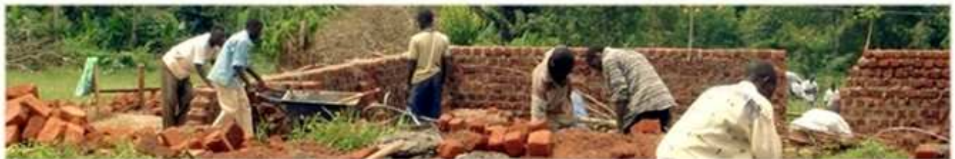
The early stages of construction of the science laboratory and kitchen at the site of 'Onwards & Upwards' School, Buloba. (August 2007)
